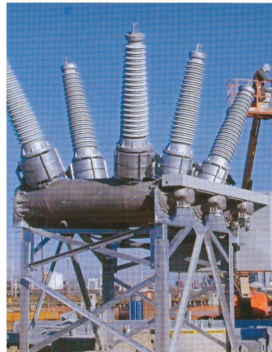
ASTORIA ENERGY POWER PLANT
